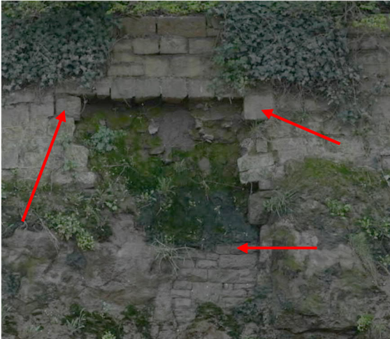
Figure 7.7: NCS13 Collapsed section 2019
