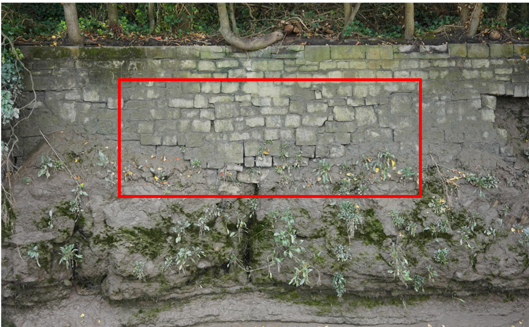
Figure 7.4: NCS13 Typical example of minor wall deformation
