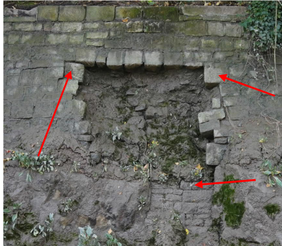
Figure 7.8: NCS13 Collapsed section 2022
