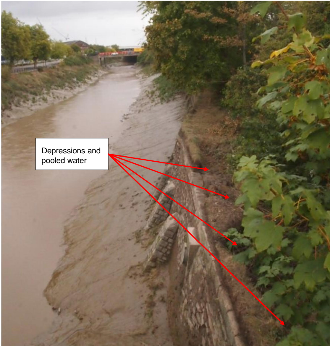
Figure 10.14: NCS28 Upstream depressions behind wall
