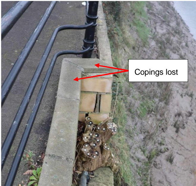
Figure 9.11: NCS21 & NCS23 Lost copings
