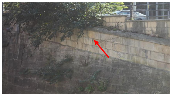
Figure 9.10: NCS21 & NCS23 Leaning wall 2022
