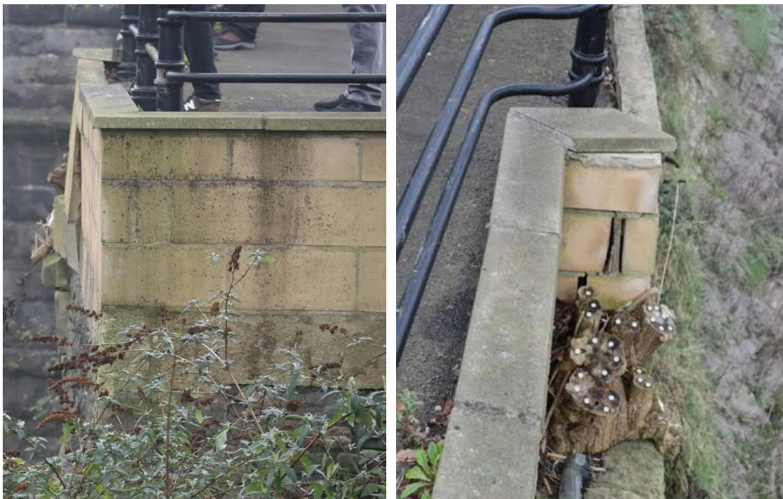
Figure 9.4: NCS21 & NCS23 Wall deformation
