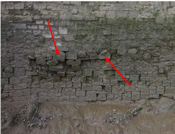
Figure 8.10: NCS18 Wall deformation 2019
