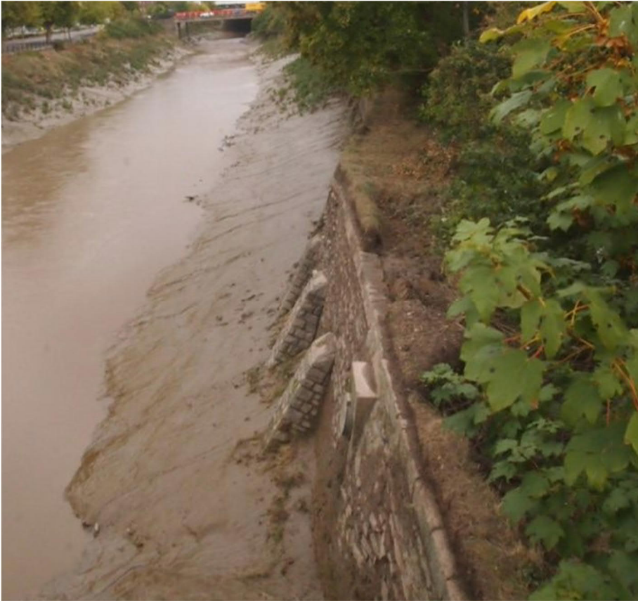
Figure 10.5: NCS28 Upstream area of deformation view from bridge
