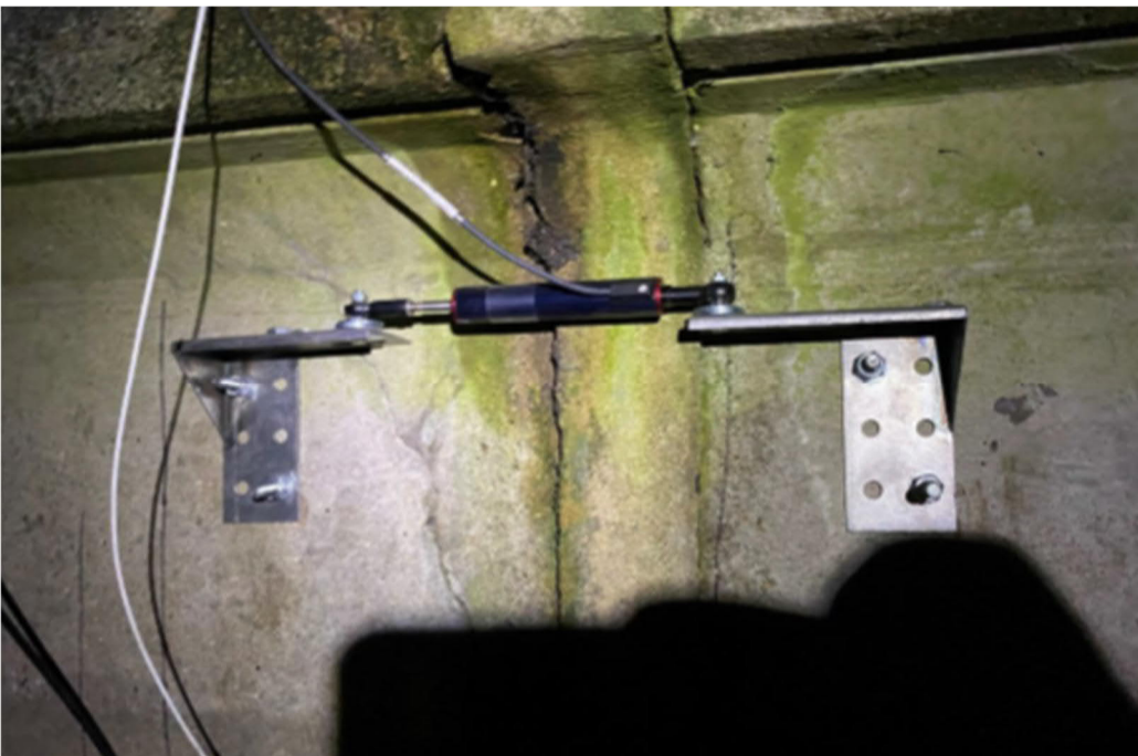
Figure 2.3: Typical linear displacement sensor across crack
