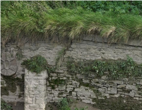
Figure 10.17: NCS28 Open joint 2019
