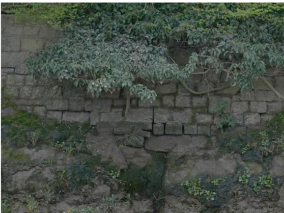
Figure 7.9: NCS13 Wall deformation 2019
