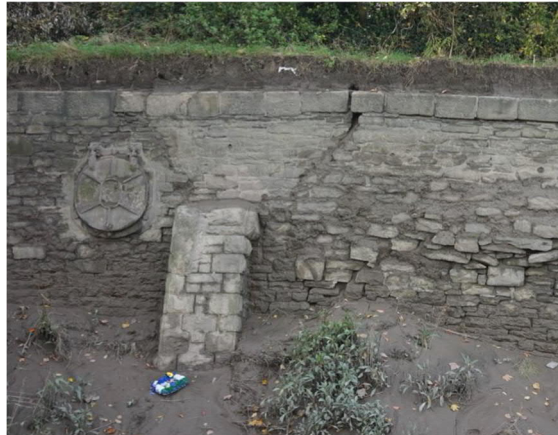
Figure 10.18: NCS28 Open joint 2022
