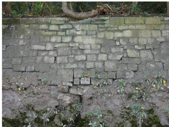
Figure 7.10: NCS13 Wall deformation 2022
