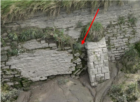
Figure 10.15: NCS28 Wall deformation 2019
